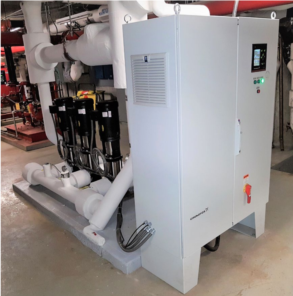
Actual Installation from the Grundfos Energy Optimization Program
